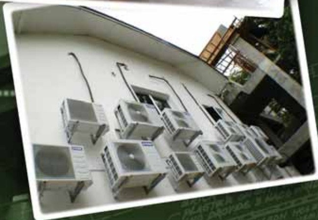
Recently installed air-conditioners spoiling the side facade
