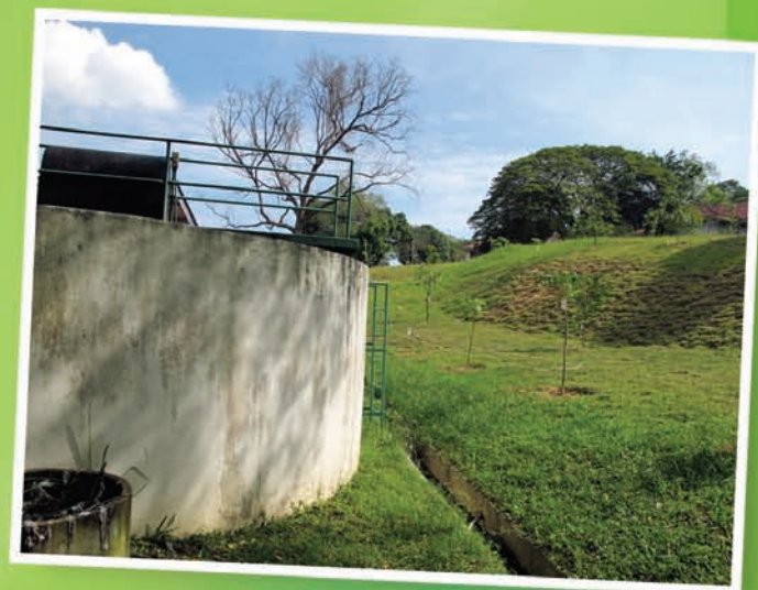
USM engineers dubbed this concrete chamber as the 'tank that washes itself'
