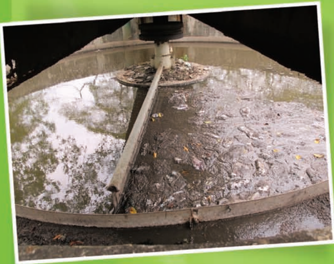
Entrapped sanitary pads inside the clarifier tank
