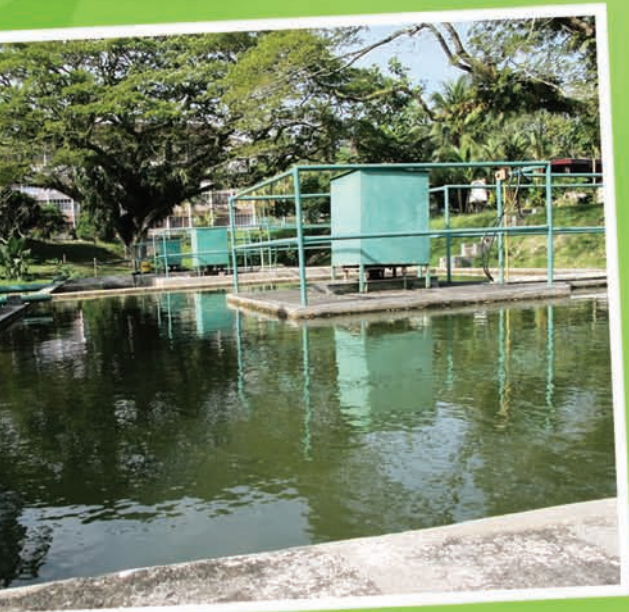
Aeration (background) and sludge holding tanks
