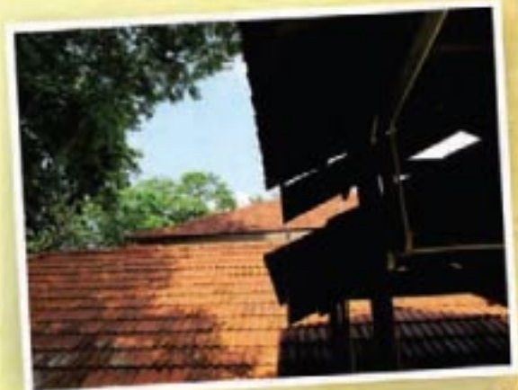
These roofs are designed for tropical weather as they drain water easily during heavy downpour
